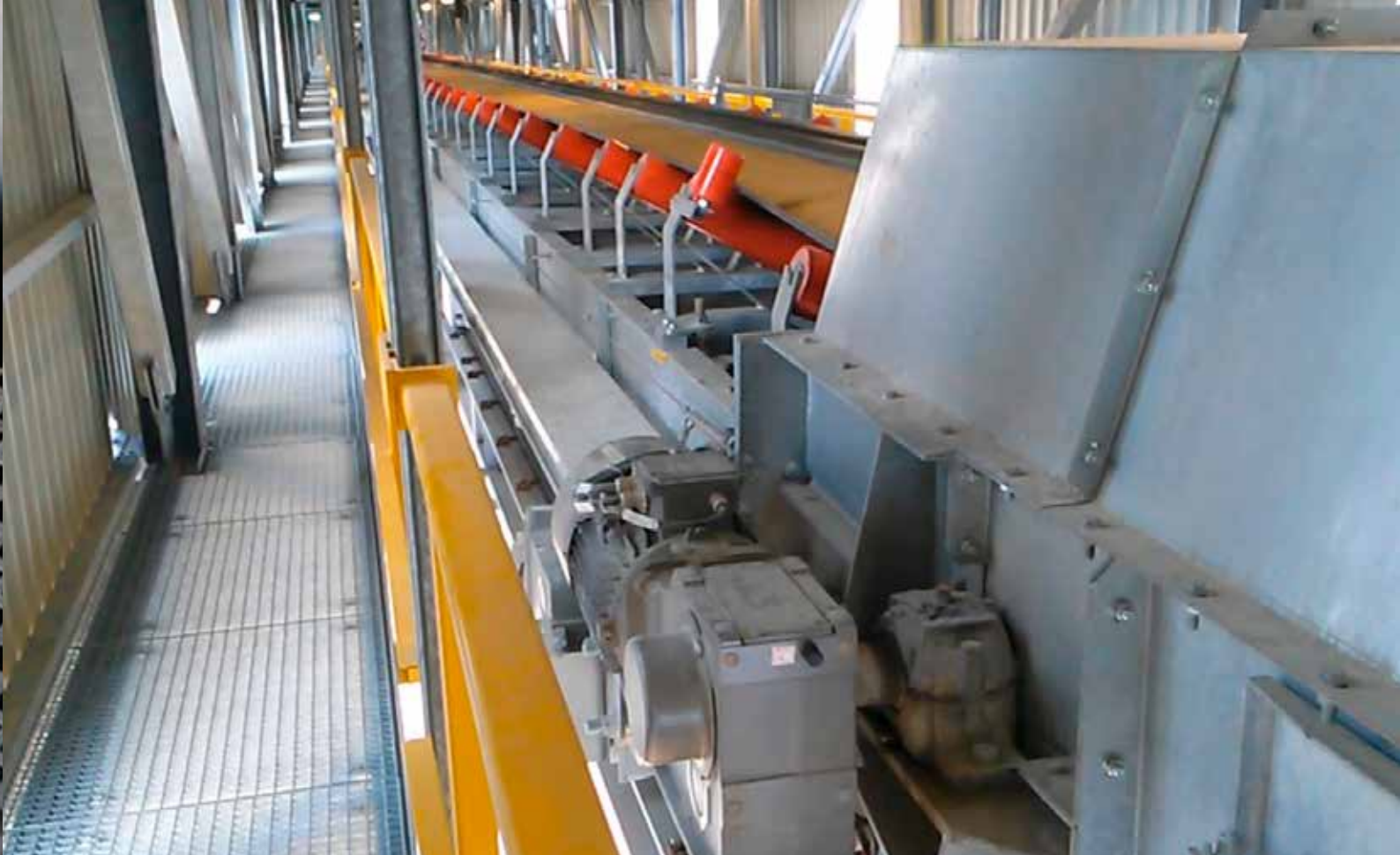
Figure 3: This conveyor belt deposits the bunker material.
